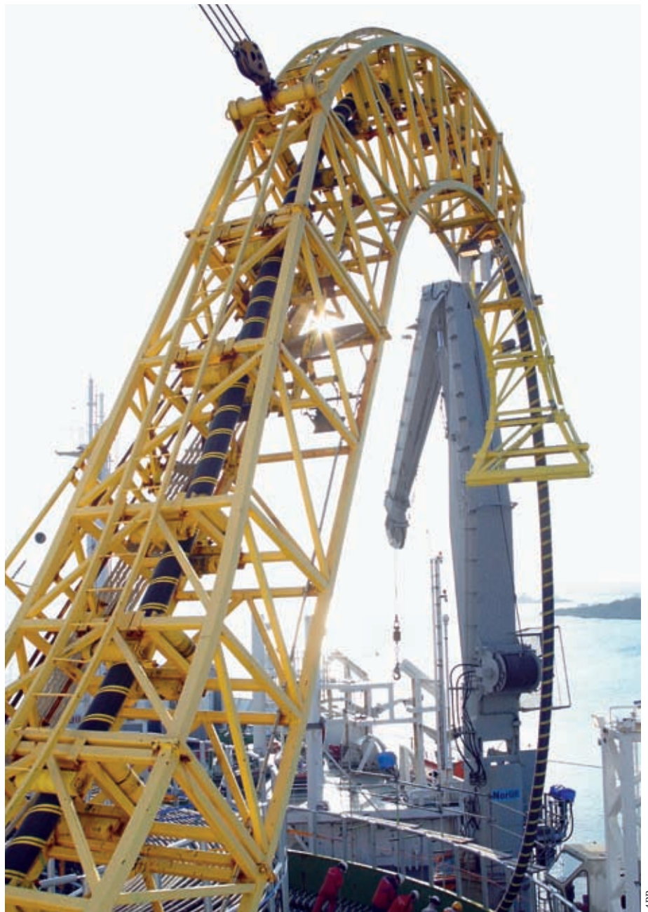
The project turnkey supplier ABB is constructing a new link to connect the Baltic countries with the EU electricity network.
